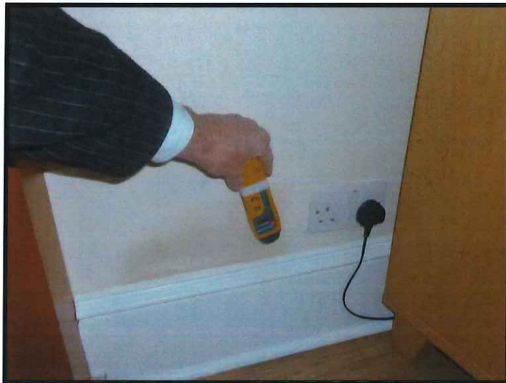
Figure 7 Lounge wall right hand side fireplace visible staining/high damp reading
