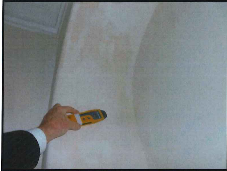
Figure 6 Lounge wall left alcove visible staining/high damp reading
