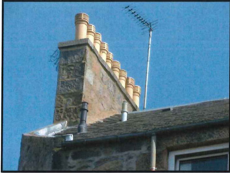
Figure 4 Rear view West Chimney - vegetation visible
