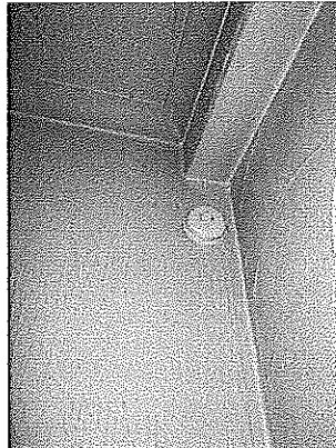
Living Room - Carbon Monoxide alarm
