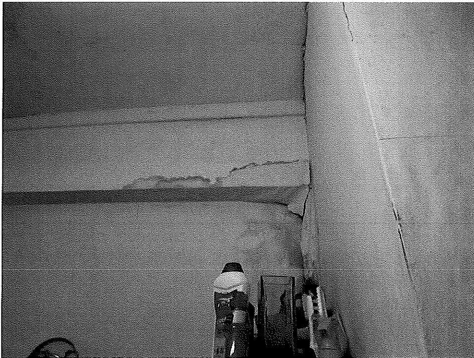
Damp staining on upper wall of Kitchen from leaking pipe
