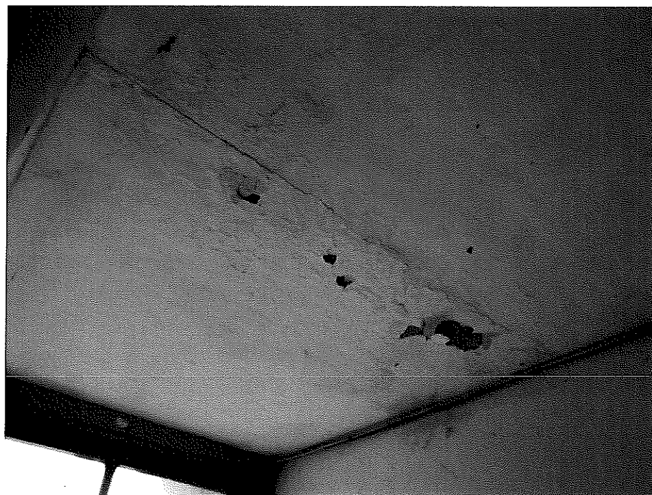
Damage to stairwell ceiling
