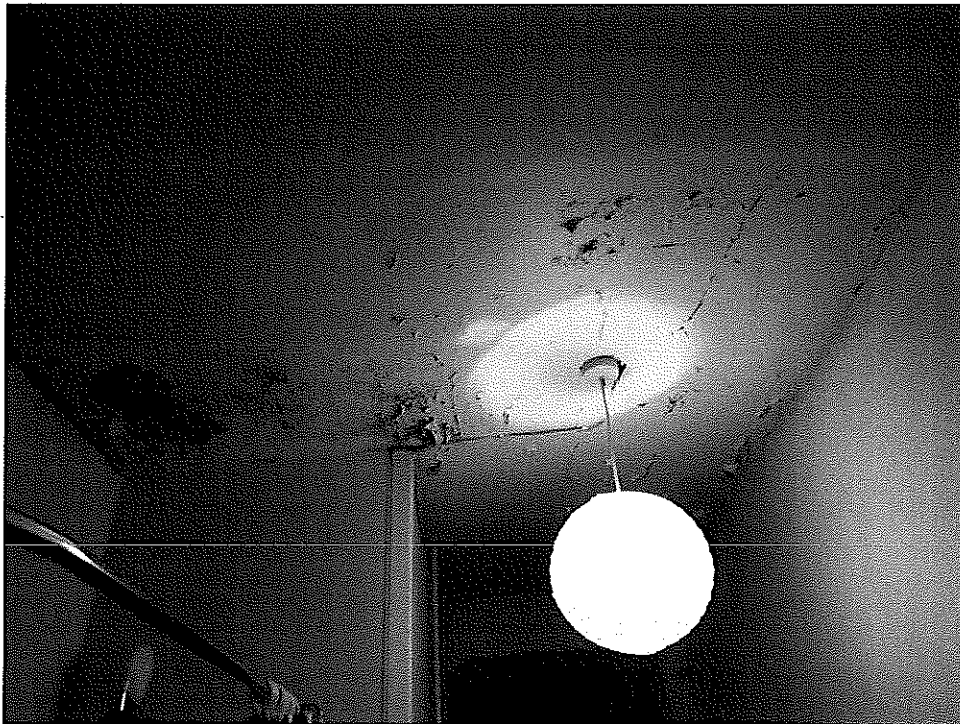
Cracked/damaged Bathroom ceiling
