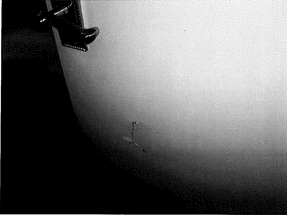
Damage to Lounge door
