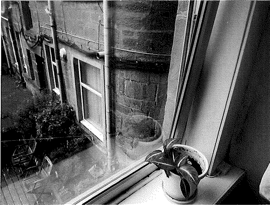
Condensation at Bedroom 1 window (Replacement window casement)
