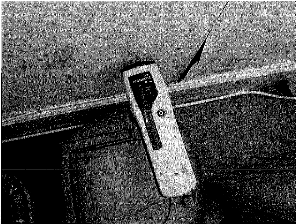
Condensation below Bedroom 1 window
