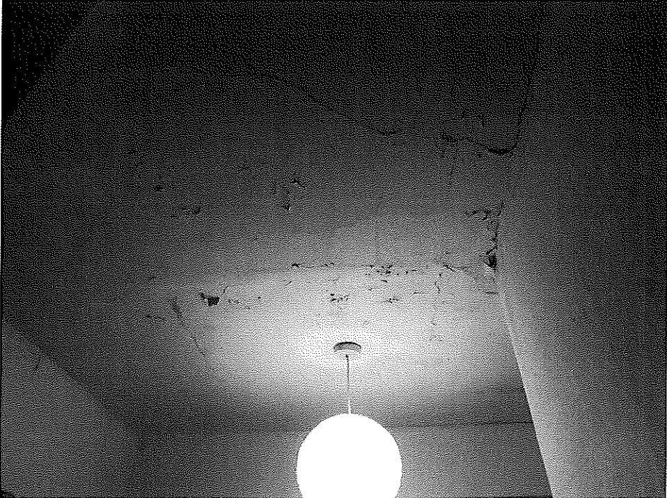
Cracked/damaged Kitchen Ceiling
