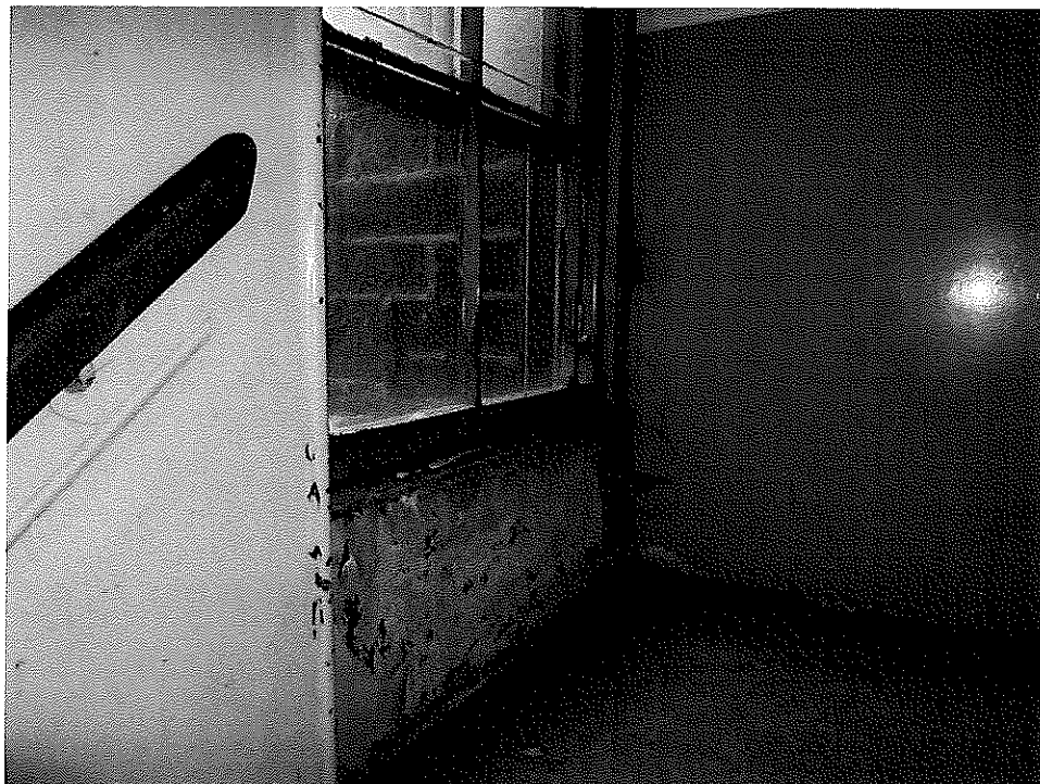
Damage to stairwell window
