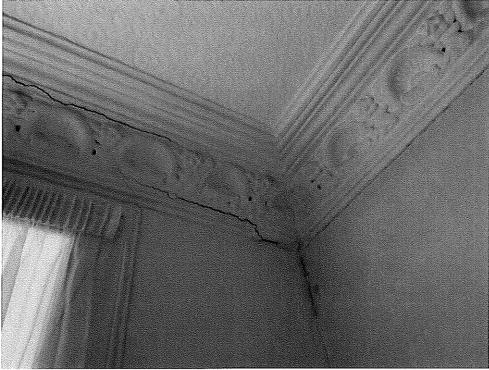
Old damp stain on upper wall in Lounge and cracking to cornice
