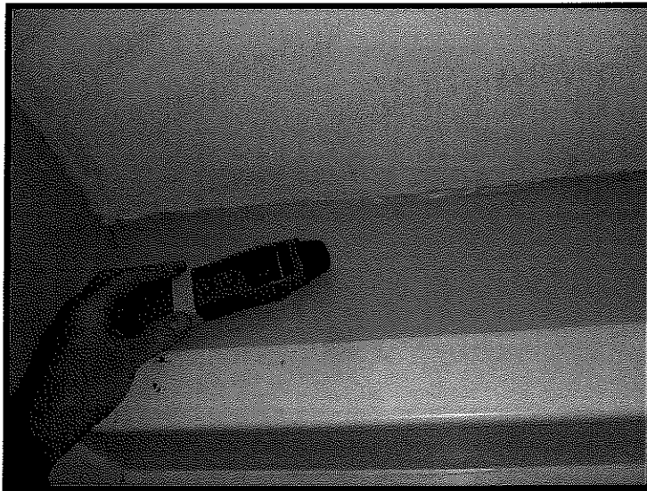
Figure 5 High dampness Lounge wall beneath shower location
