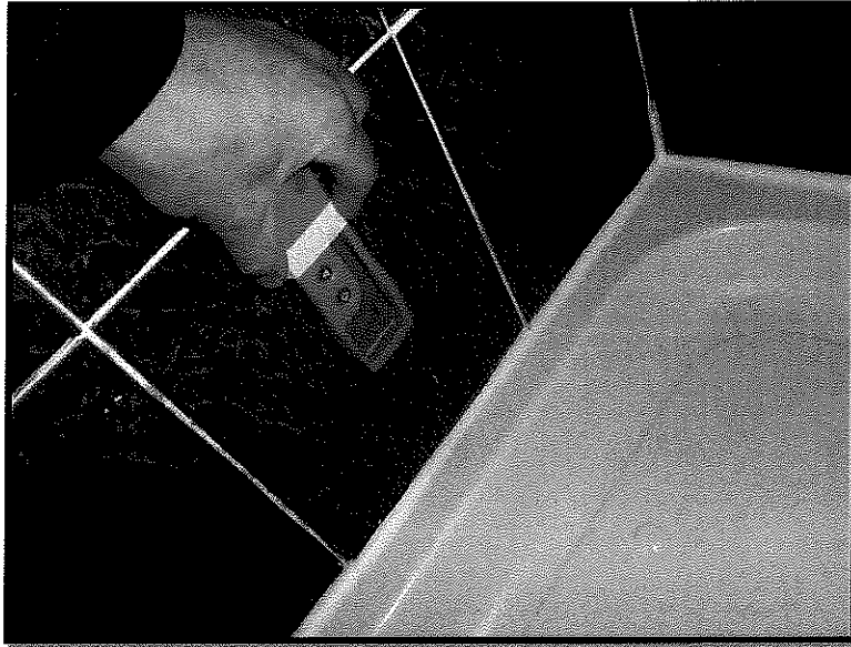
Figure 8 High dampness shower enclosure
