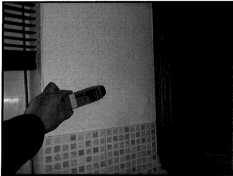
Figure 3 Moderate dampness Kitchen wall (front)
