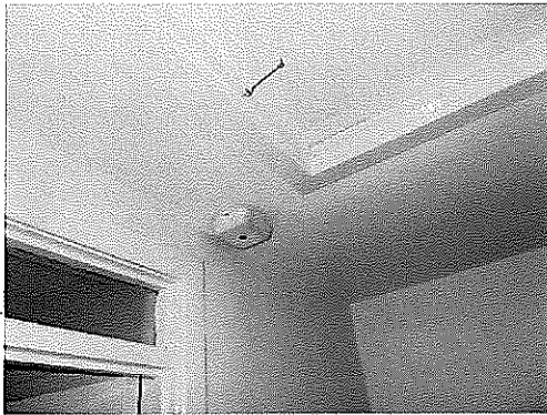
Battery Smoke alarm landing
