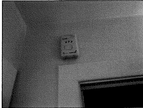
New Carbon Monoxide alarm on wall outside cupboard in front vestibule
