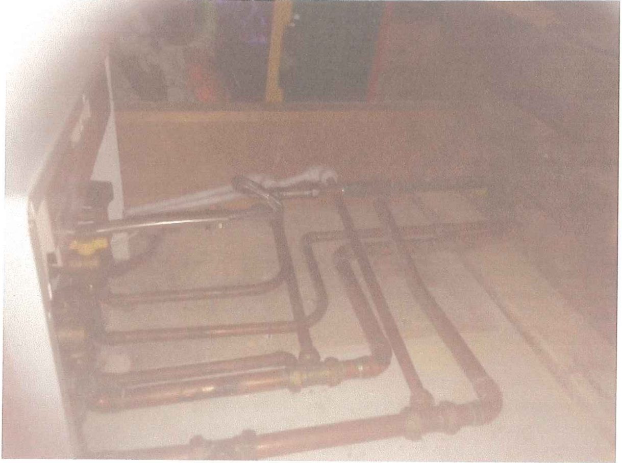
10. A shower has been installed in what appears to be a former cupboard which forms part of the bathroom
