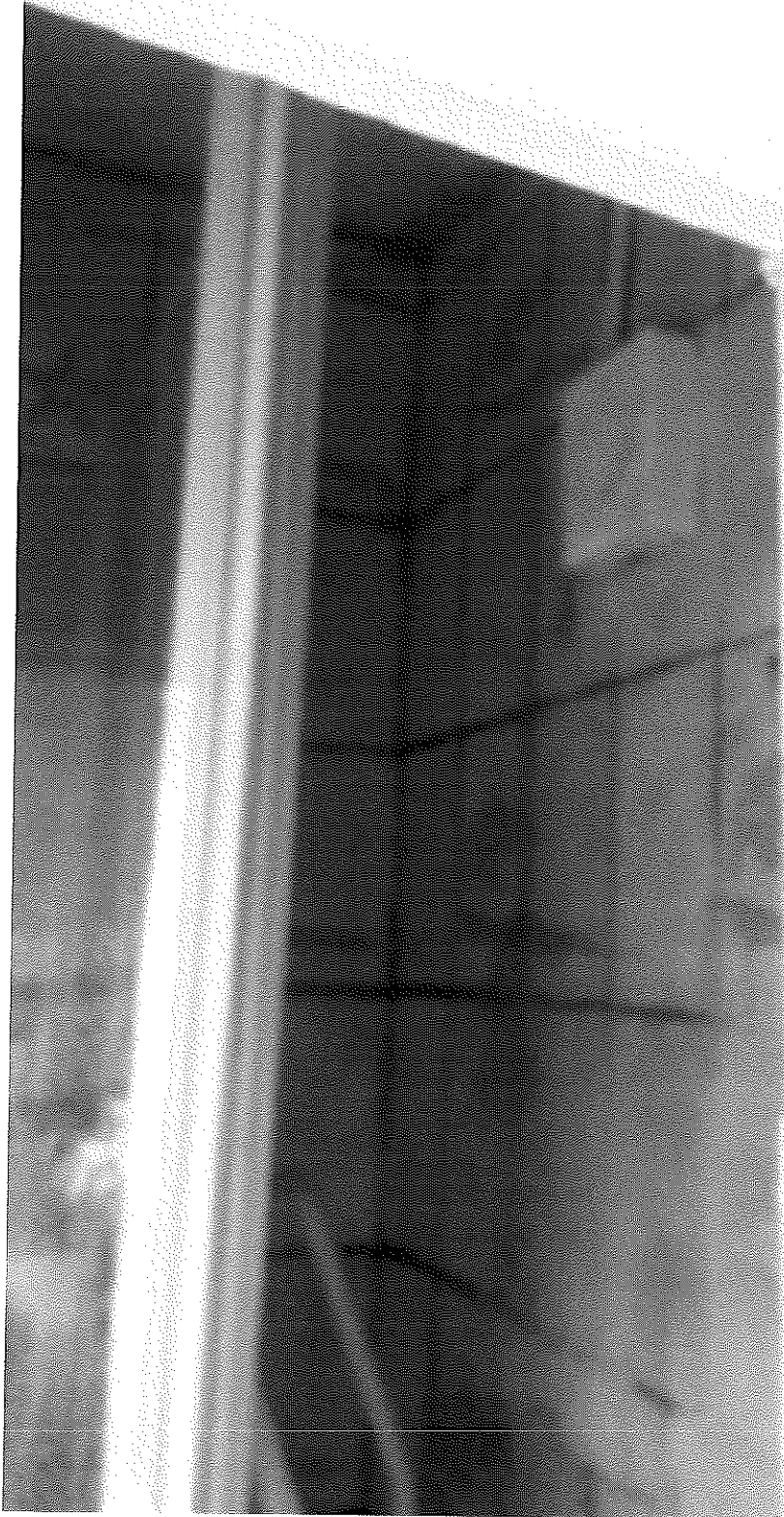
13. There is no operable extractor fan in the shower area
