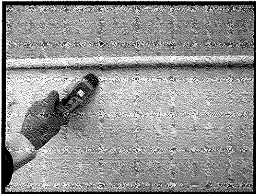
Figure 9 Rear Bedroom Ceiling Damp Reading
