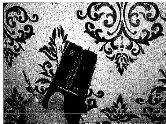
Damp reading- bath wall
