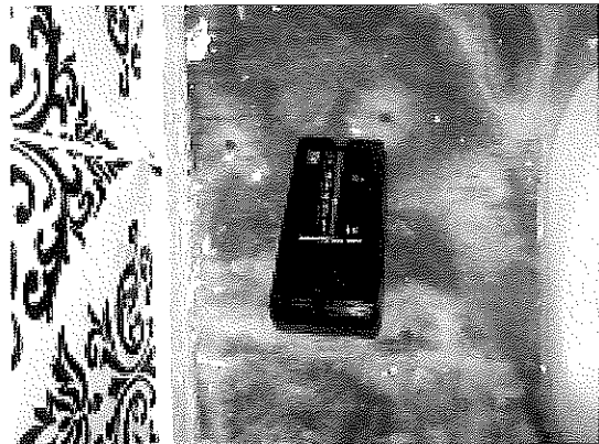
Damp reading-bath floor
