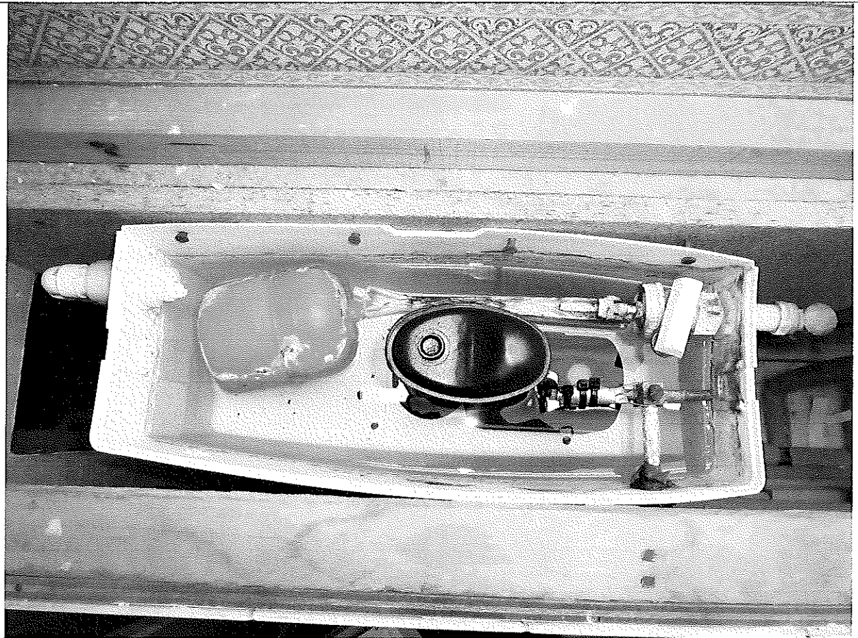
Temporary repair to cistern and blocked overflow pipe on the left
