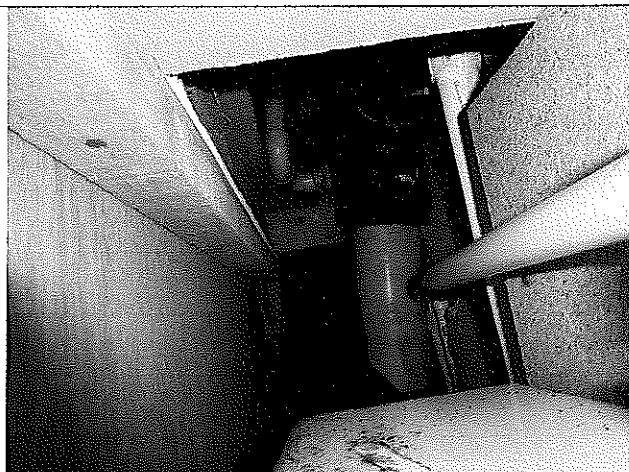
Wet floor behind toilet
