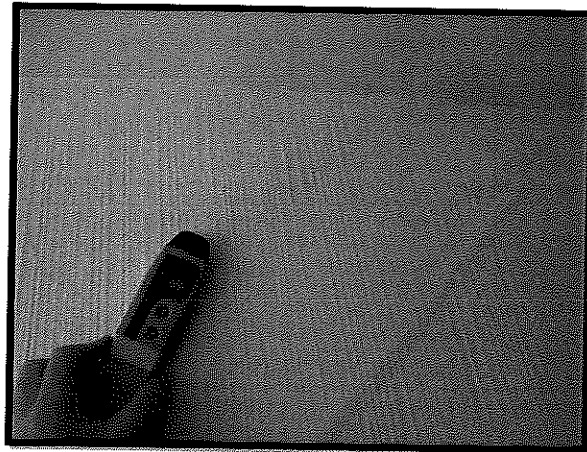
Figure 9 Main Bedroom Damp Reading
