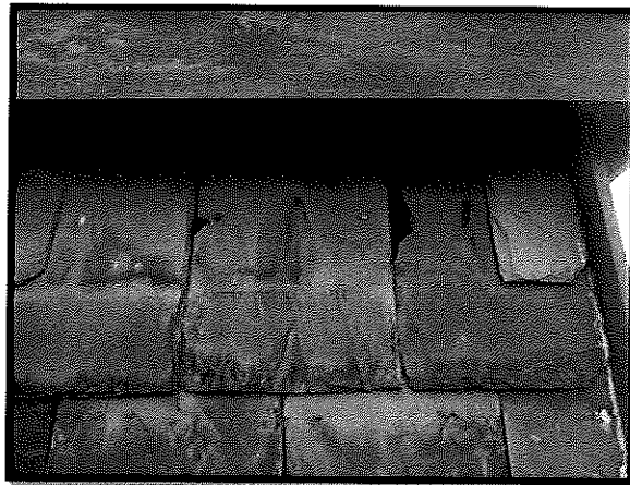
Figure 11 Missing slates at dormer
