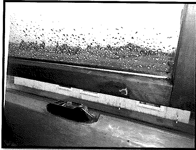
Figure 7 Example of missing or broken handles
