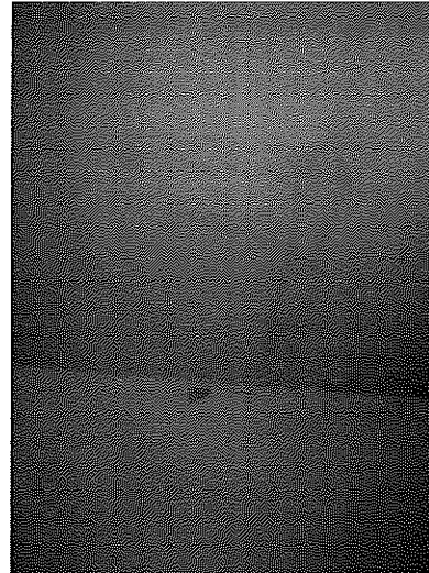
Living Rm—stain on ceiling
