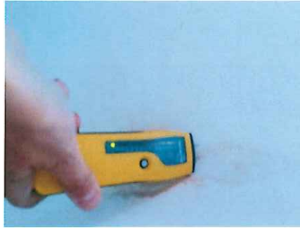
Dampstaining to living room
