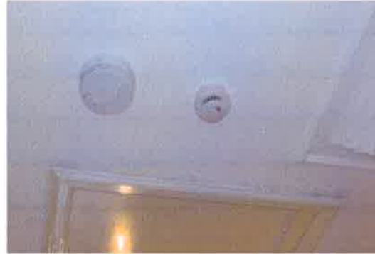
(Ph12) Stairwell ceiling smoke detector
