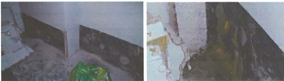
(Ph1) FE – Basement Bedroom L/H/S (Ph2) FE – Basement Bed. Extreme L/H/S
