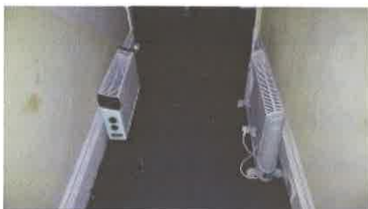
(Ph23) Moveable electric heaters
