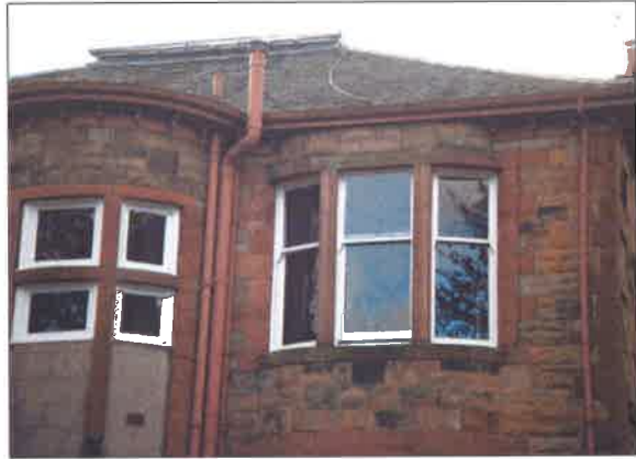
Rear elevation - Roof condition poor
