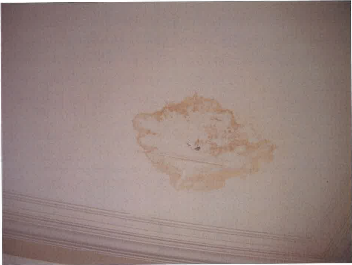
Dining room - Historic water ingress
