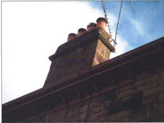
Gable - Chimney crown weathered
