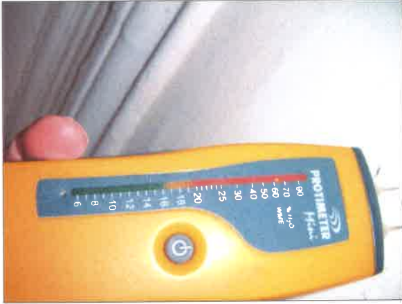
Lounge – water ingress and carpet staining
