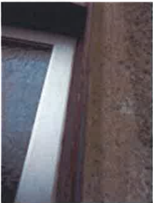
External Kitchen door showing sealant
