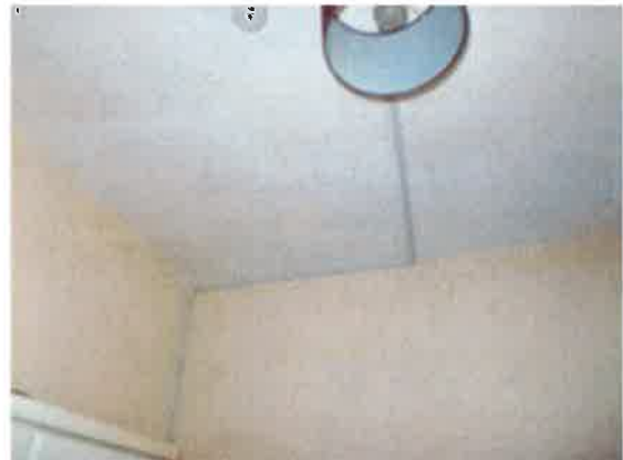
Kitchen - pendant light fitting
