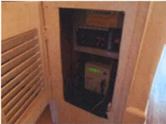
Hall - fuse box
