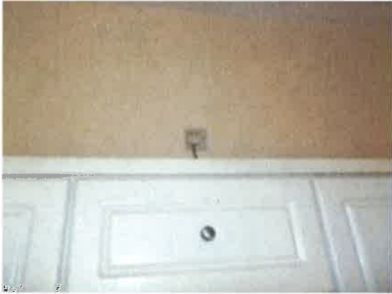
Kitchen - socket above kitchen units
