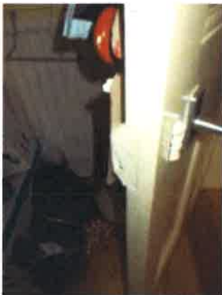
Front Bedroom Door - jammed/missing bolt
