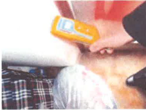
Kitchen - wall to left hand side of external door - high moisture reading at base
