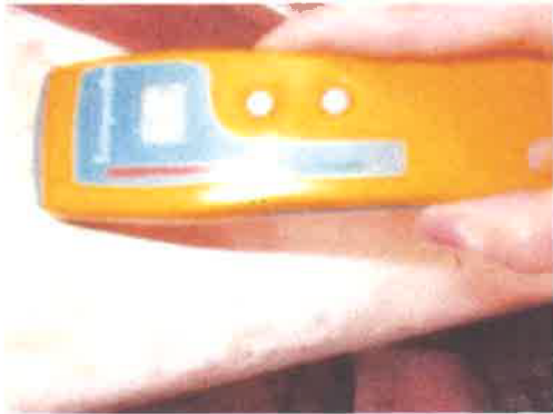
Kitchen - wall to left hand side of external door - high moisture reading at damp patch
