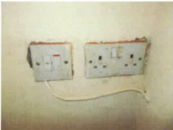
Kitchen - double socket and switch - exposed electrical cable and damaged plaster.
