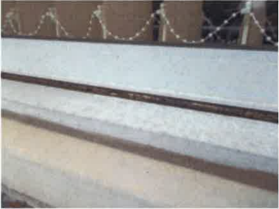
Living Room - bay window - external perished seal
