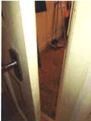
Kitchen Door - jammed/missing bolt
