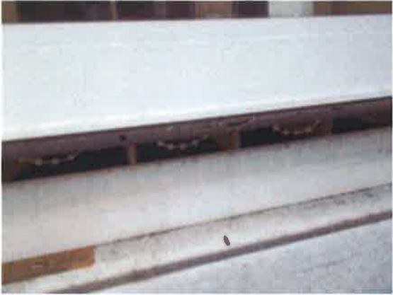
Living Room - bay window - external perished seal
