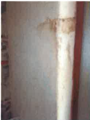
Kitchen - wall to left hand side showing damp patch
