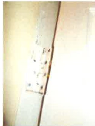
Bathroom Door- loose hinges
