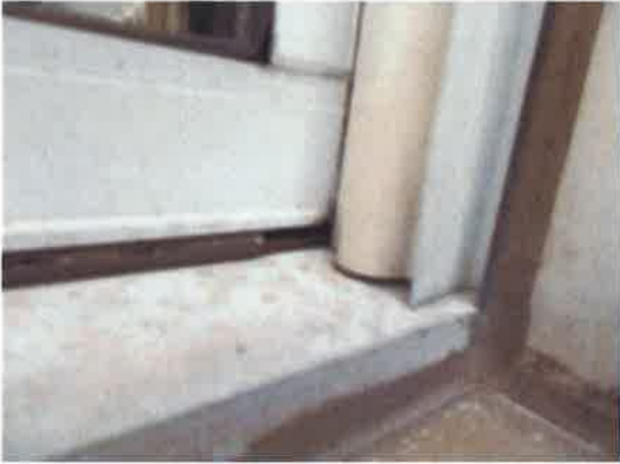
Living Room - bay window - external perished seal and gap
