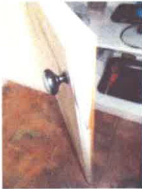
Kitchen - base unit door to left side of oven - outer coating peeling
