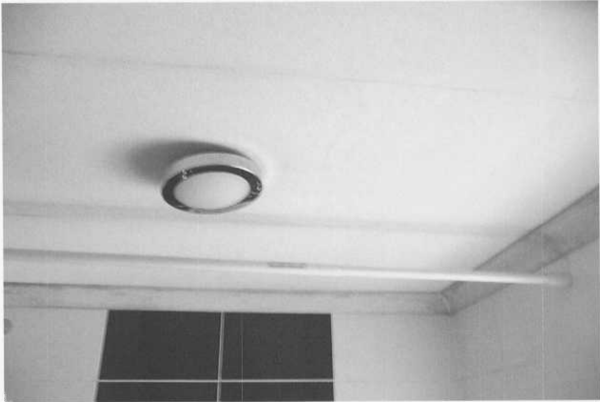
Bathroom ceiling – note discolouration of coving
