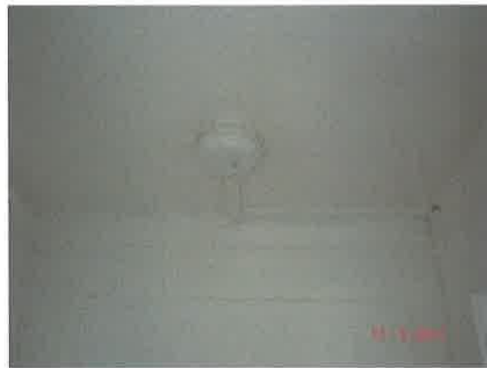
SMOKE DETECTOR – HALL
