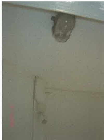
LIGHT AND PIR SENSOR-TOP FLOOR
