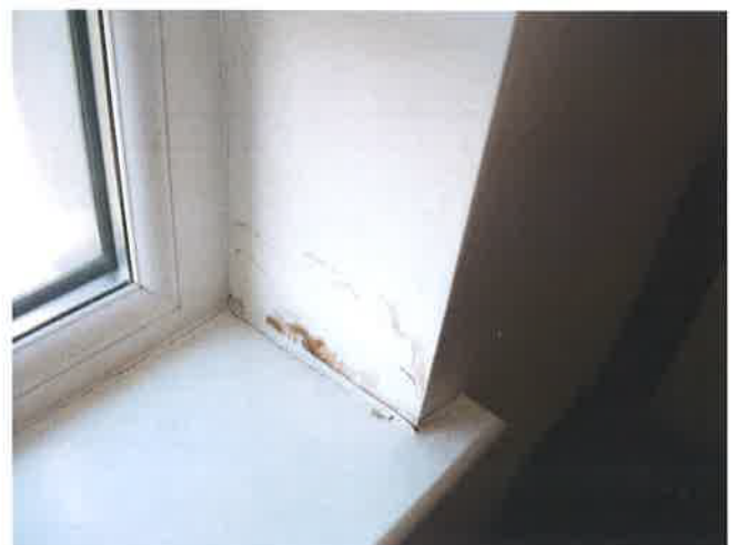
07 - Bedroom RHS showing water damage
