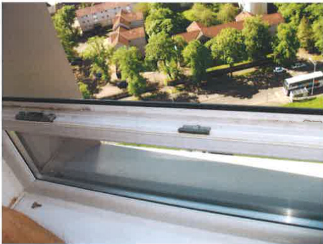
04 - Internal drains slots enlarged
