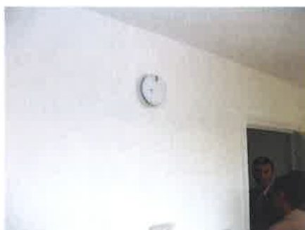
14 – Mains smoke alarm (Living room)
