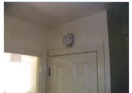
15 – Mains smoke alarm (Hall)
