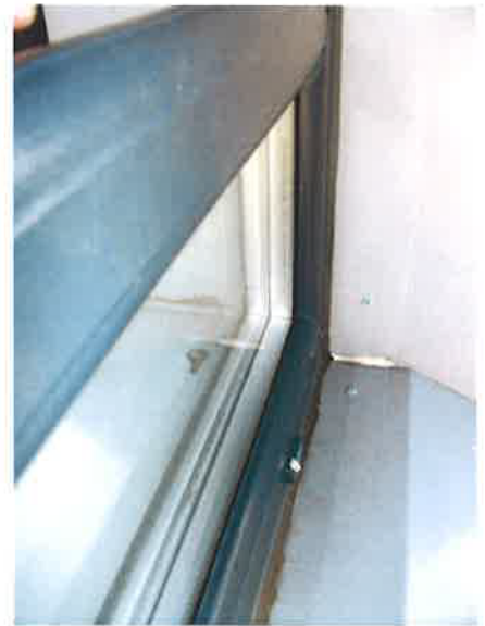
03 - External drain outlet & cover
