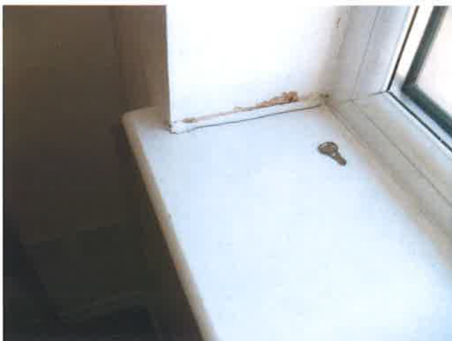
06 - Bedroom LHS showing water damage
