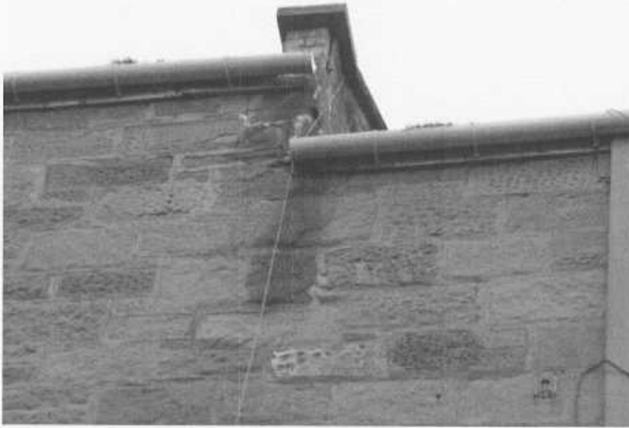
Choked rear gutter
