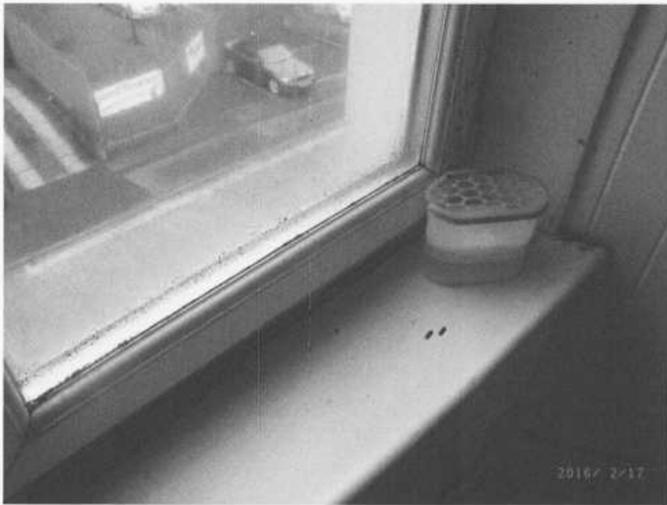
Dampness at Lounge window
