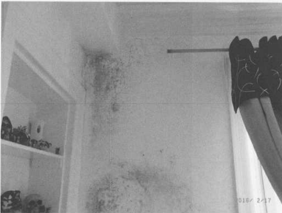
Typical dampness/mould in Lounge
