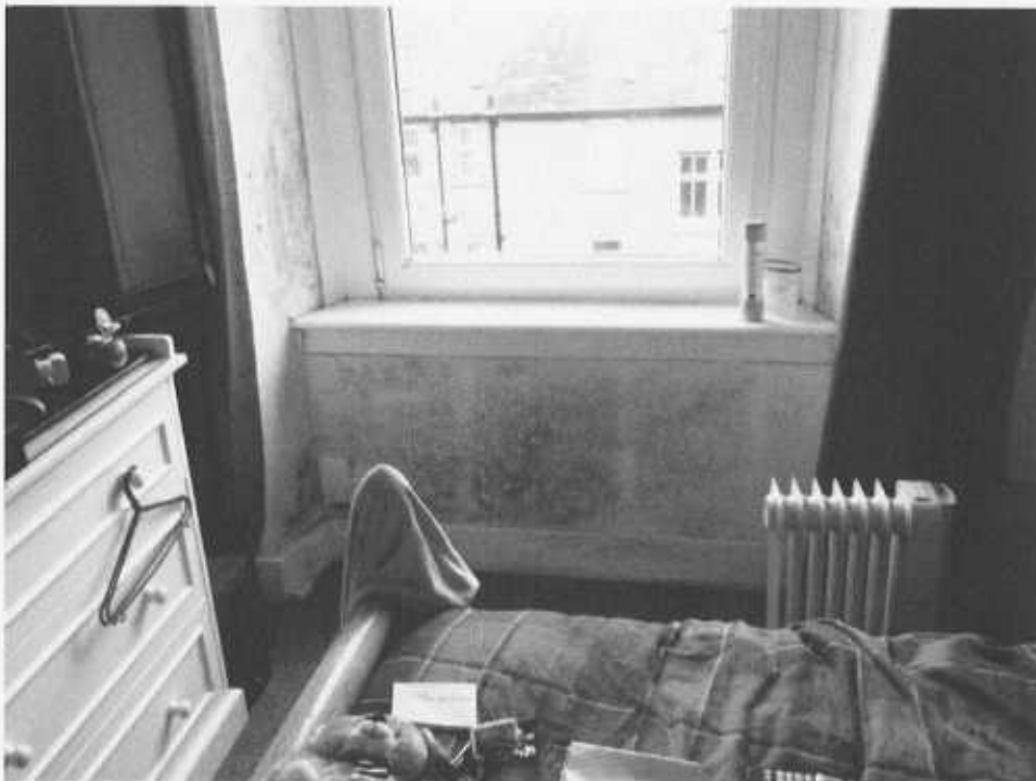
Typical dampness/mould in Bedroom
