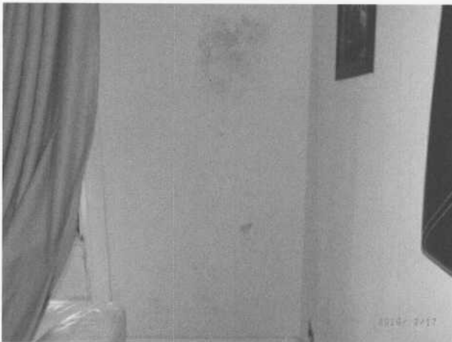
Typical dampness/mould in Lounge
