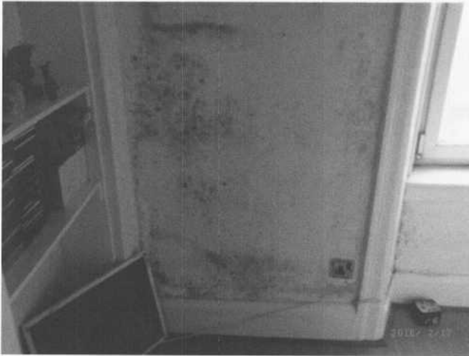
Typical dampness/mould in Lounge
