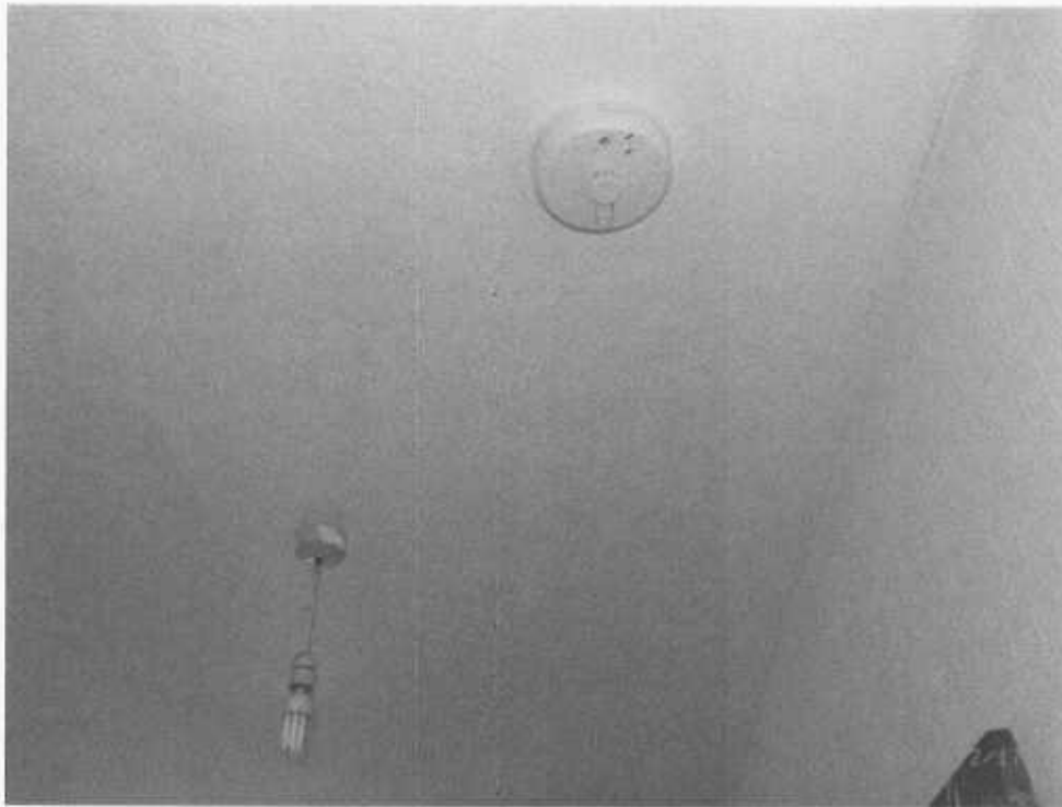
New heat detector in Kitchen
