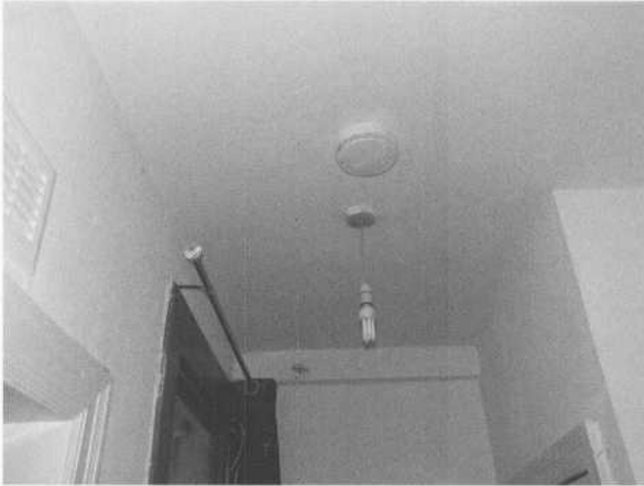
New smoke detector in Hall
