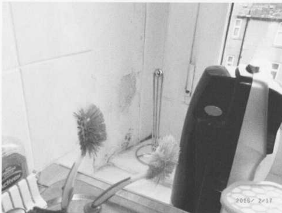
Typical dampness/mould in Kitchen
