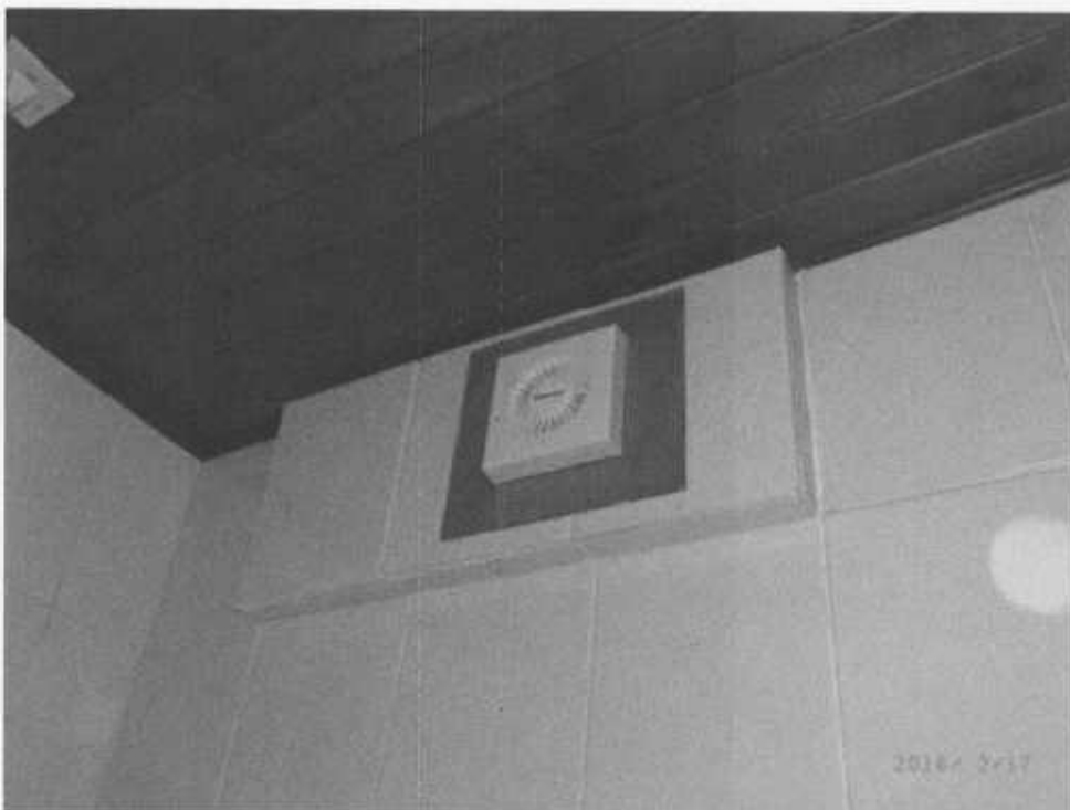
Ventilator in Bathroom
