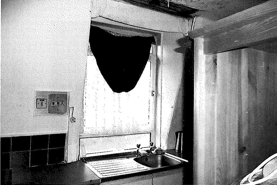
Kitchen window – does not fully close
