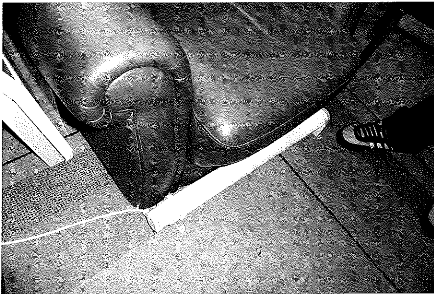
Rail heater found by tenant in loft not fixed to floor/wall
