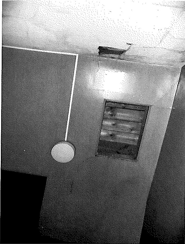
Former roof light boarded and slated over
