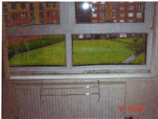
Distorted window frame in Bed
