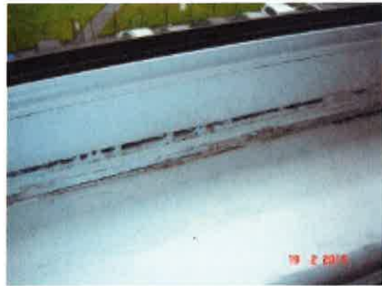
Gap in frame
