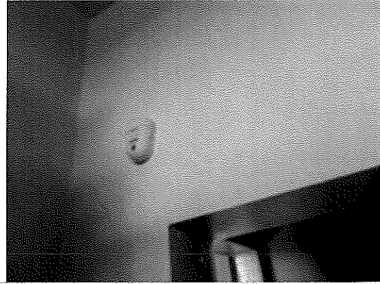
Kitchen - Wall mounted CO alarm
