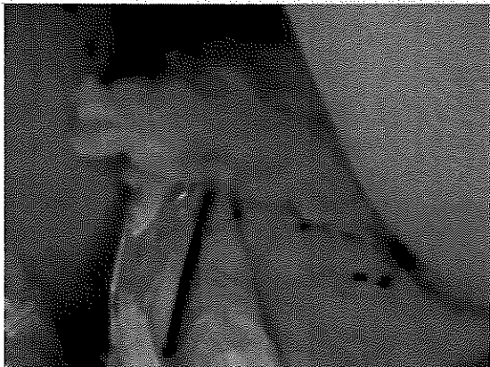
Bathroom - space under bath - evidence of rodent activity
