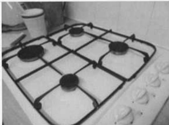
Gas Hob in Kitchen
