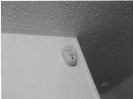
Carbon Monoxide Alarm in Kitchen
