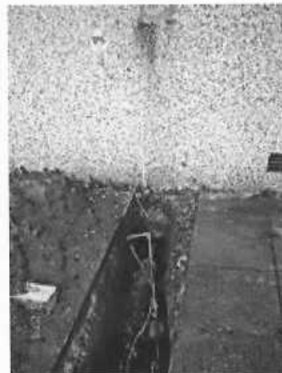
New/old feed supply For central heating
