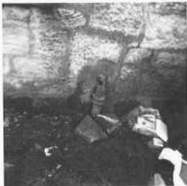
17. Kitchen Sink Waste Externally
