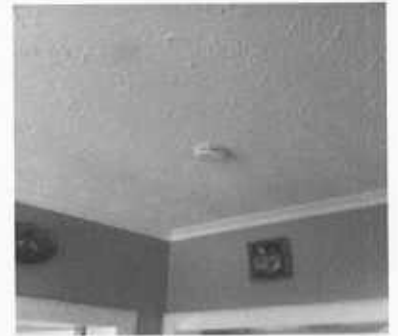
10. Battery Smoke Alarm GF Hall
