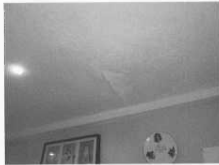
9. Water Damage Kitchen Ceiling
