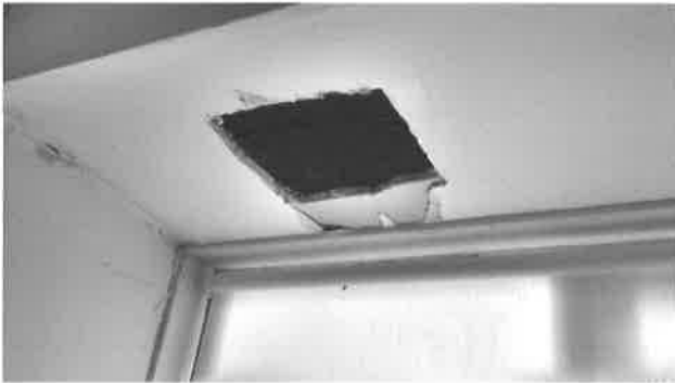
3a) As at 26/04/16: hole in kitchen ceiling under bathroom
