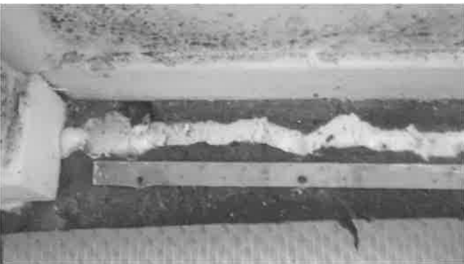
2a) As at 26/04/16 showing mildew
