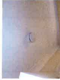
7. Hard wired smoke detector dining room
