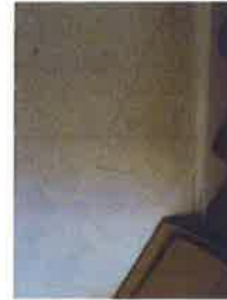
4. Cracking to artex on stair
