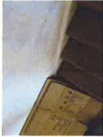
5. Cracking to artex on stair
