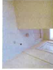
9. Hard wired smoke detector hall
