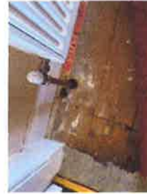
3. Holes at Living Room radiator
