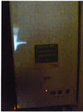
5. Central Heating Boiler
