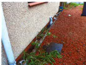
11. Broken Rodding Point Cover
