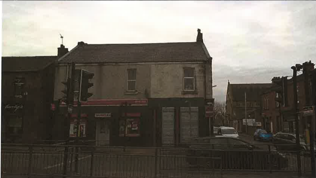
1B Hozier Street. Front elevation. Roof has been completely retiled, new leadwork and new guttering
