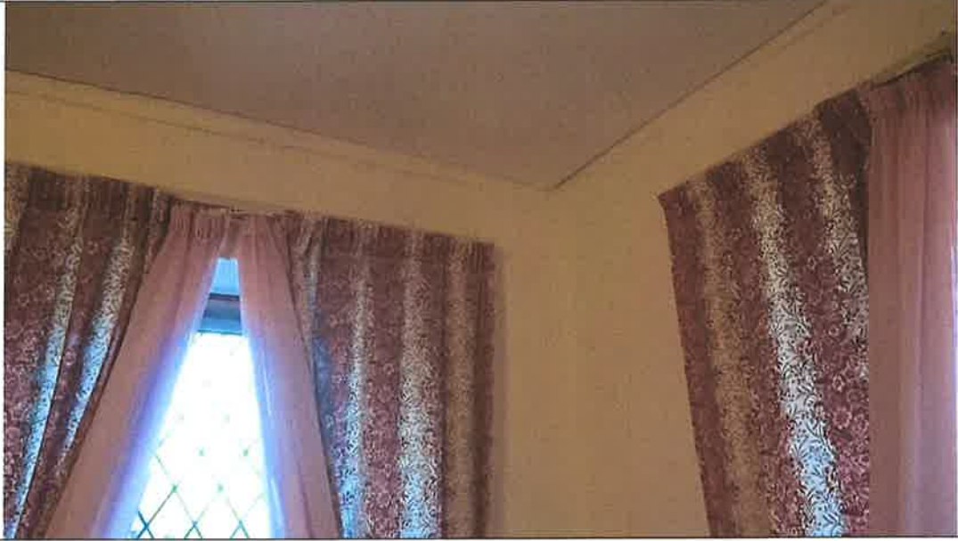
Bedroom has been redecorated following repair of roof. High damp readings found adjacent to bottom of windows, may be related to defective pointing and harling.
