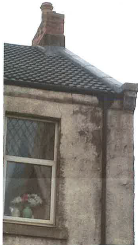
Front elevation. Harling and pointing remains in poor condition.
