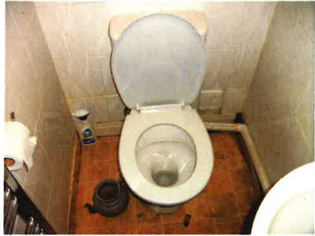
28 - WC & WHB (under the stairs)
