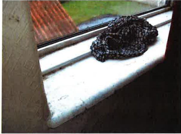
08 – Stair window (water on sill)
