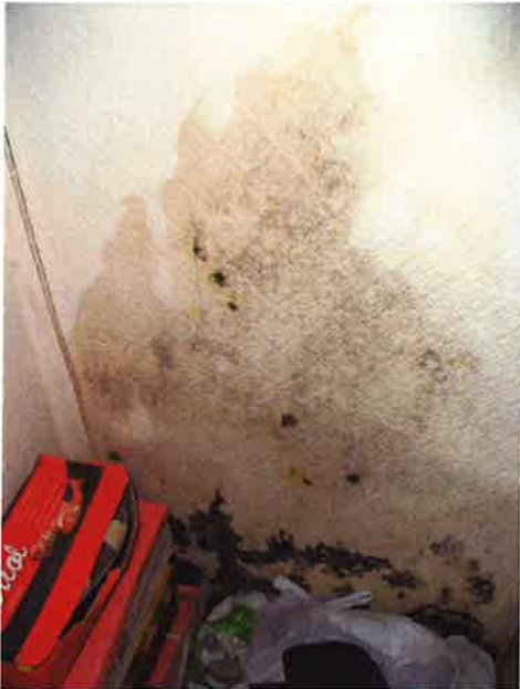
23 – Rear Bedroom (severe dampness on wall)
