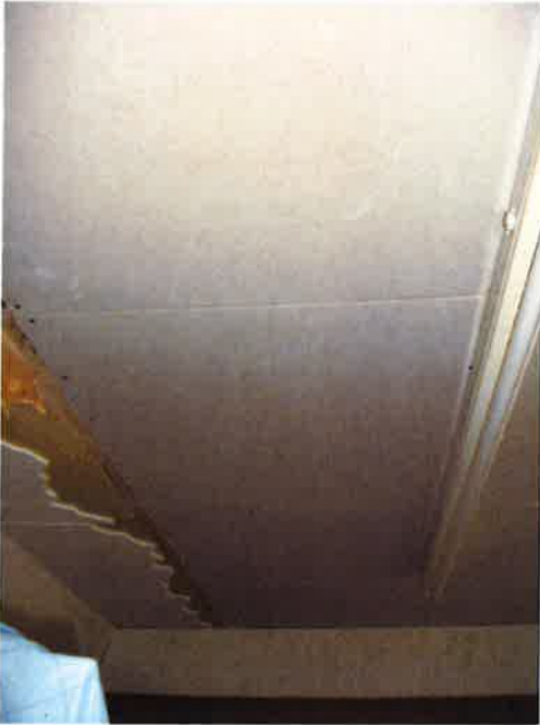
01 – Kitchen ceiling (temporary repairs)
