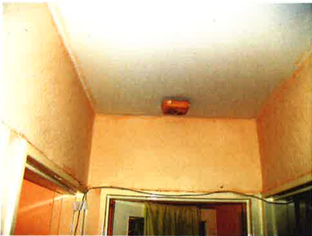
29 – Lower hall - battery operated smoke detector
