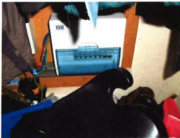
26 – Main electricity board
