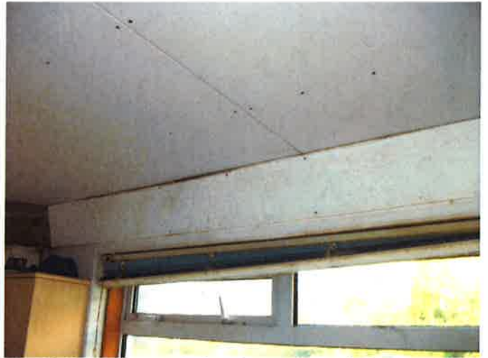
02 – Kitchen ceiling at window (temporary repairs)
