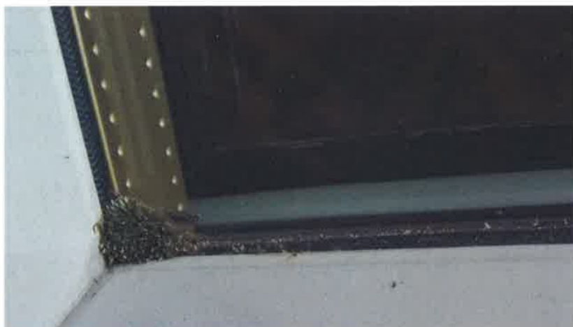
8) Living room: double glazing unit with moss growth
