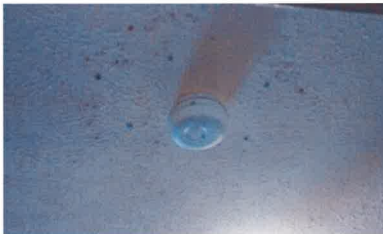
17) Heat detector: Kitchen
