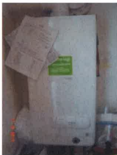
Gas central heating boiler in Kitchen
