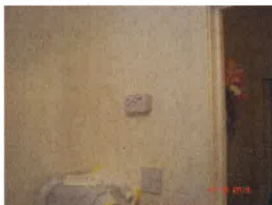
Carbon monoxide alarm in Kitchen
