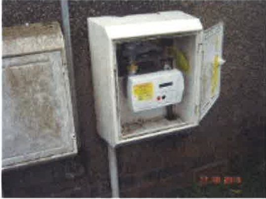
Gas meter in external cupboard.
