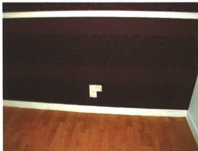
04 - Living room - power socket
