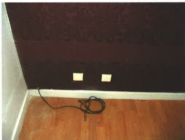
03 - Living room - power socket and TV socket
