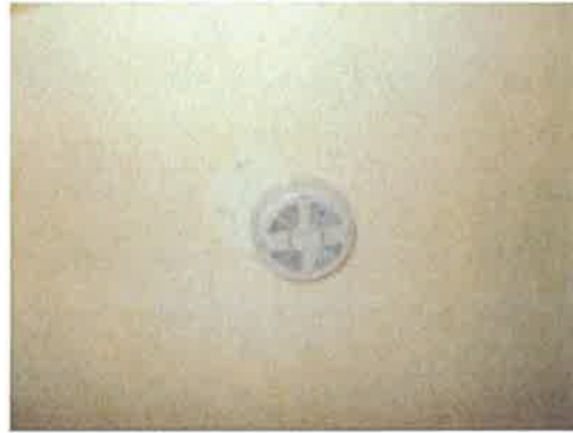
Living Room - smoke alarm
