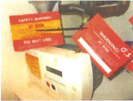
Gas Meter - 2 warning labels
