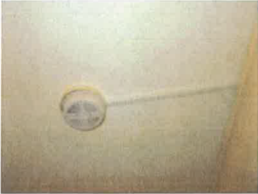
Hall - smoke alarm
