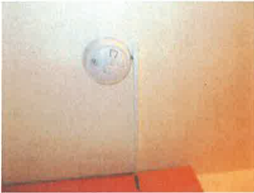
Kitchen - heat detector
