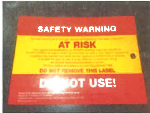
New warning label on Gas Meter
