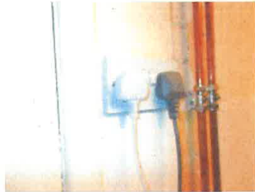
Kitchen - double socket on left side wall
