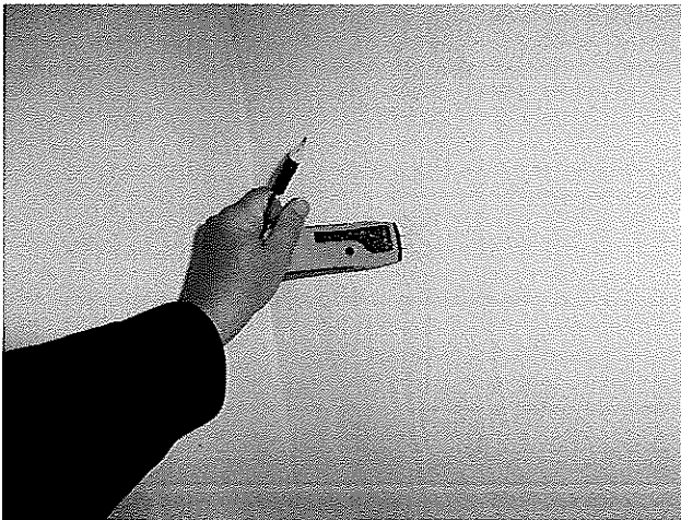
Damp meter reading 27 th May 2015
