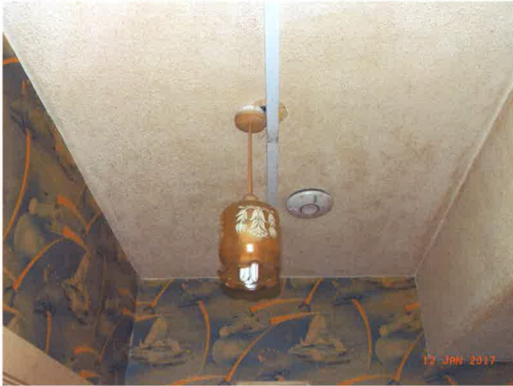
Battery powered smoke alarm in Hall
