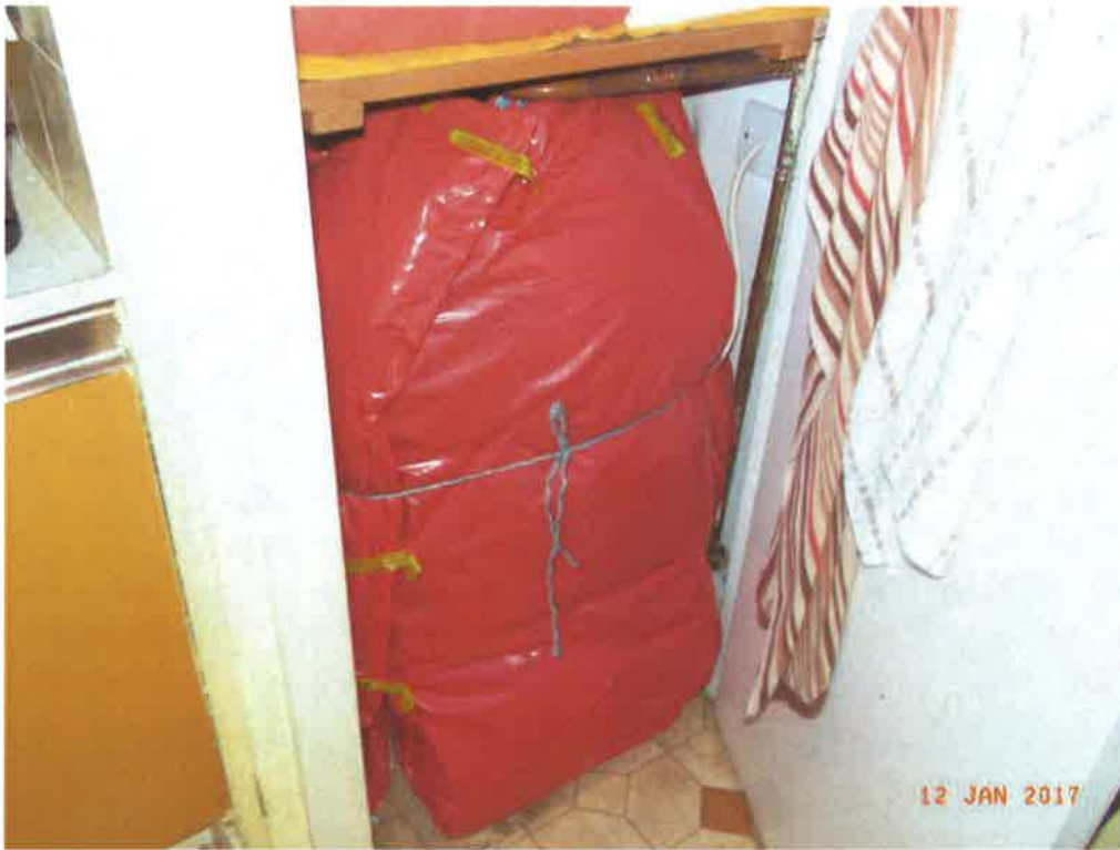
Hot water tank
