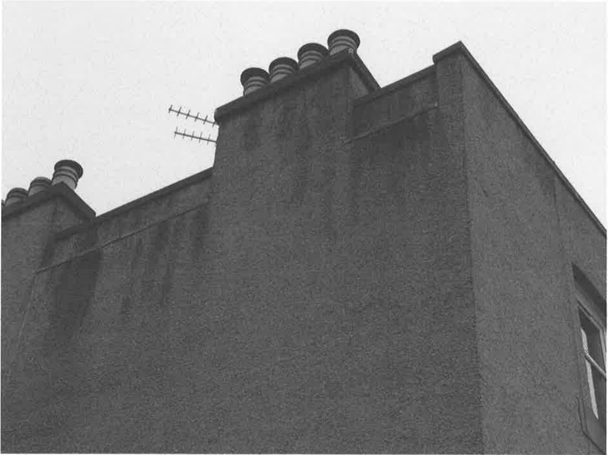
View of the gable end of the property showing the high level lead flashing RHS
