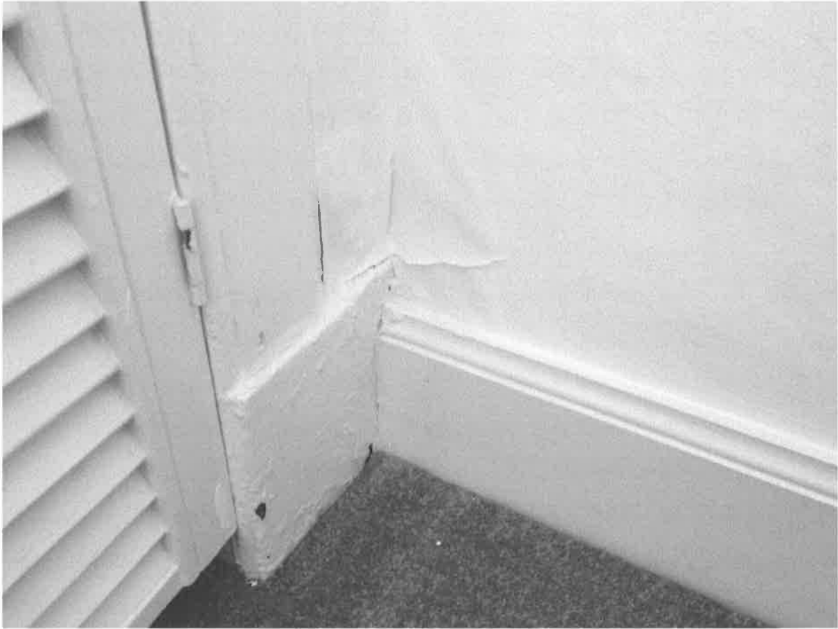
View of the peeling wall covering at skirting level in the rear bedroom as a result of historic damp penetration
