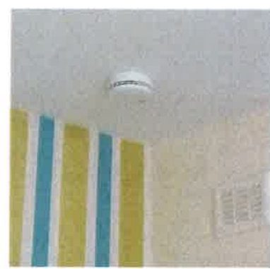
Smoke alarm in sitting room
