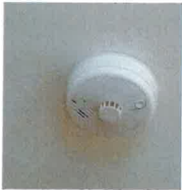
Heat alarm in kitchen
