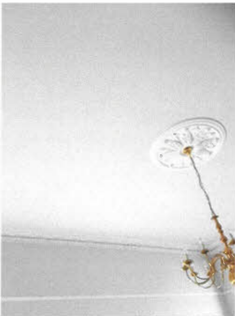
Living room ceiling - no smoke detector
