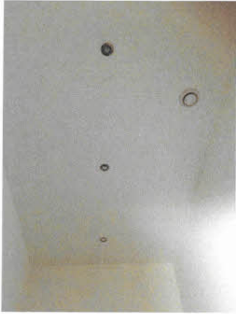
Kitchen ceiling - no smoke detector
