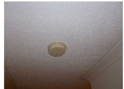
13. Battery Smoke Alarm - Hall
