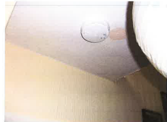
04 - Smoke detector - living room
