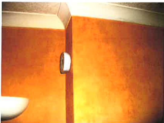
07 - Carbon monoxide detector - living room
