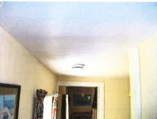
05 - Smoke detector - upper hall
