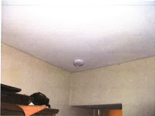
03 - Smoke detector - sitting room
