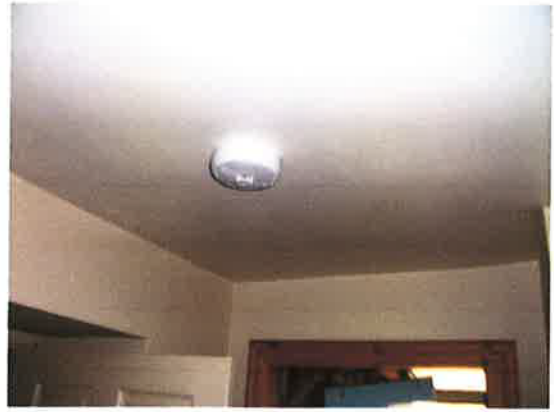
02 - Heat detector - kitchen
