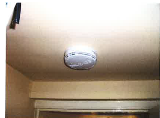
06 - Smoke detector - upstairs room
