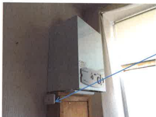
Detector fitted next to boiler in kitchen
