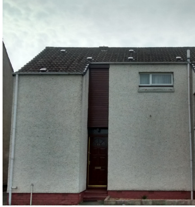
Photo 1. Front elevation showing ventilators installed in roof
