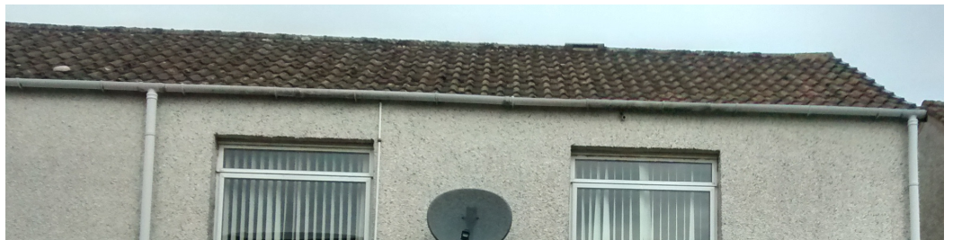
Photo 2. Rear elevation – the lower row of roof tiles has been raised and verge tiles replaced.
