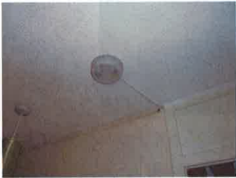
8. Hard wired smoke alarm
