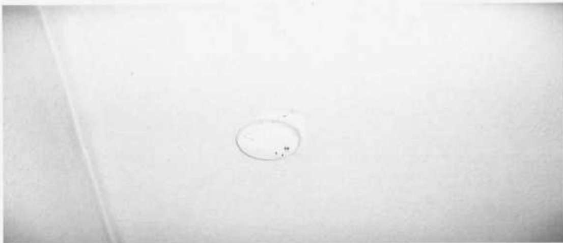
Single smoke alarm in hallway
