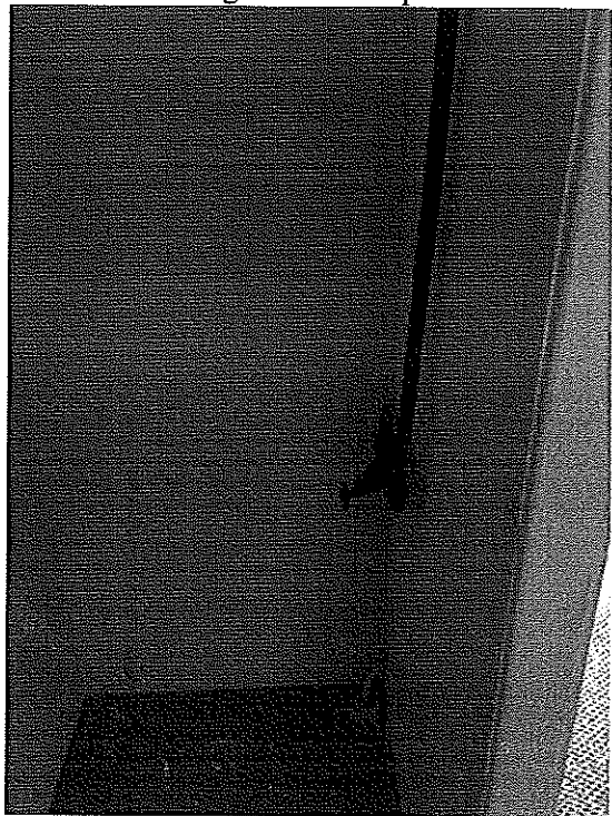
Photo 7 showing the new stopcock
