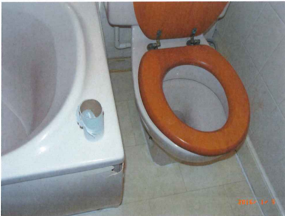
Damage to side panel of bath and loose toilet seat
