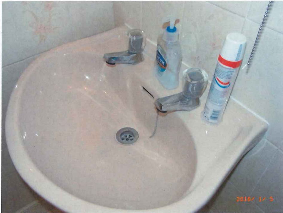
Replacement hot water tap adjacent to wash hand basin
