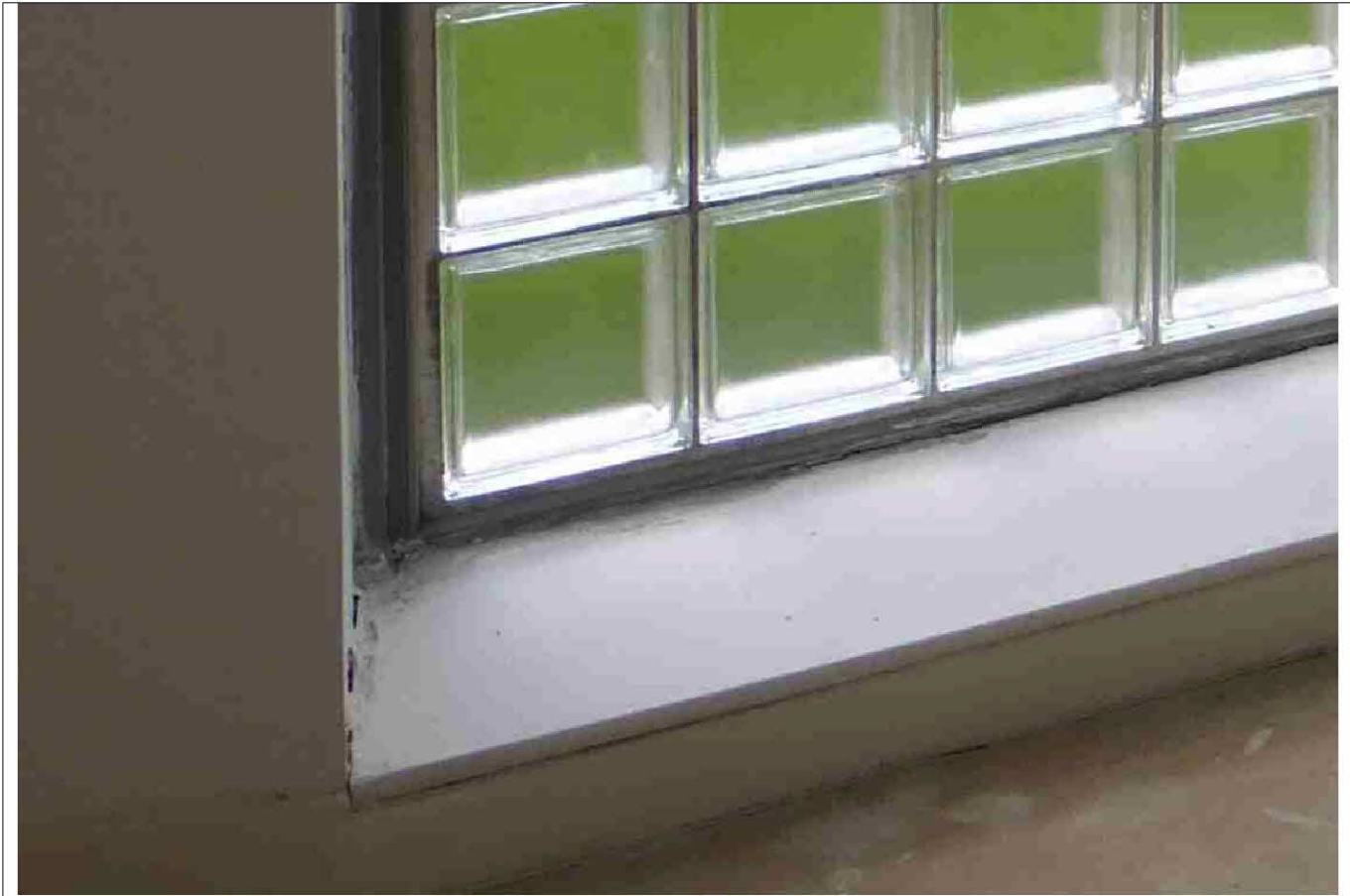
Detail of mould staining and gaps in mastic
