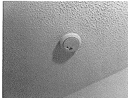
Existing smoke alarm
