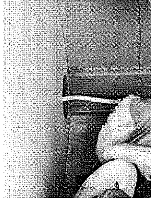
Extension wire emerging from behind unit – near front door
